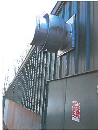
Ventilation at Woodbrook reservoir
