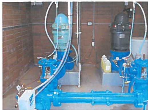
Ostrander pump station
