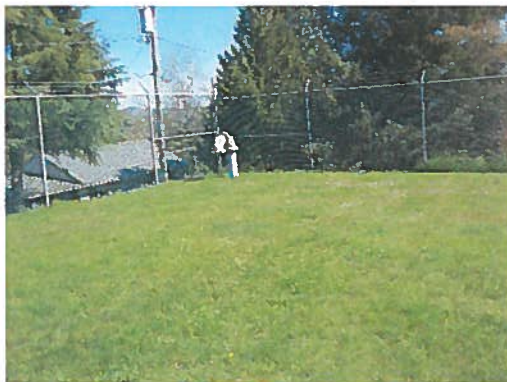
Skyline reservoir vents
